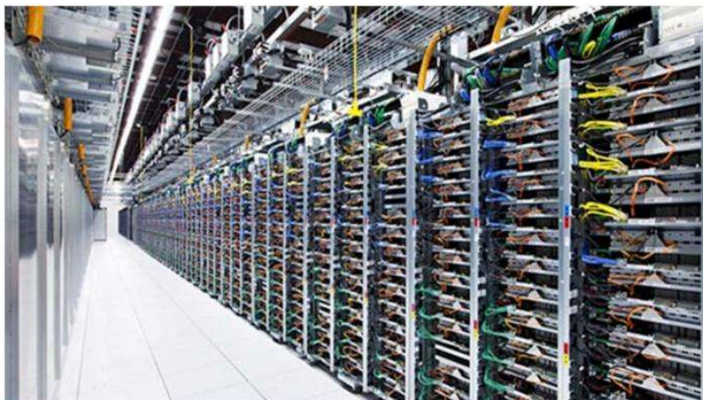
Figure 6.7 Row of server racks in a Google WSC. Although hard to see, there are bus ducts above the racks that distributed 400 V power to the servers. This picture shows a cold aisle that operators use to service the equipment.
