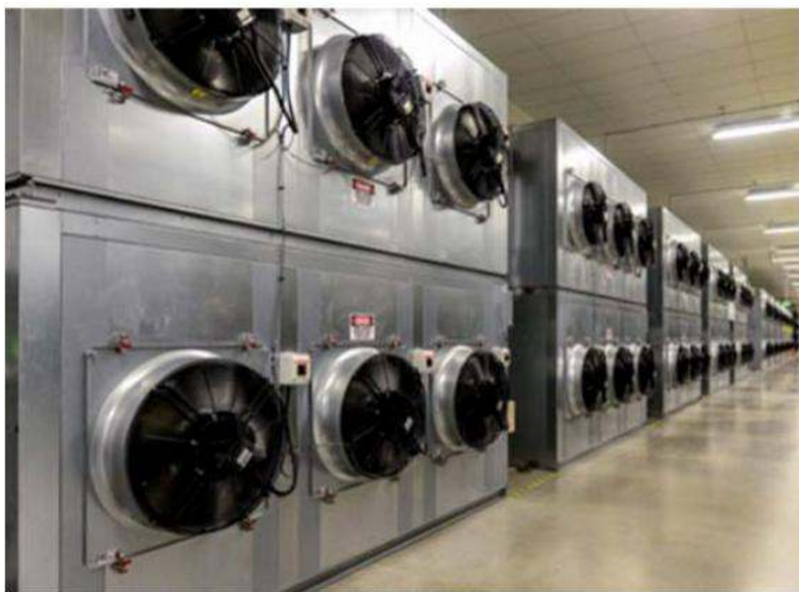
Figure 6.30 The cool air blows into the room containing the aisles of servers in a Google WSC. The hot air goes through large vents into the ceilings, where it is cooled before returning to these fans.
