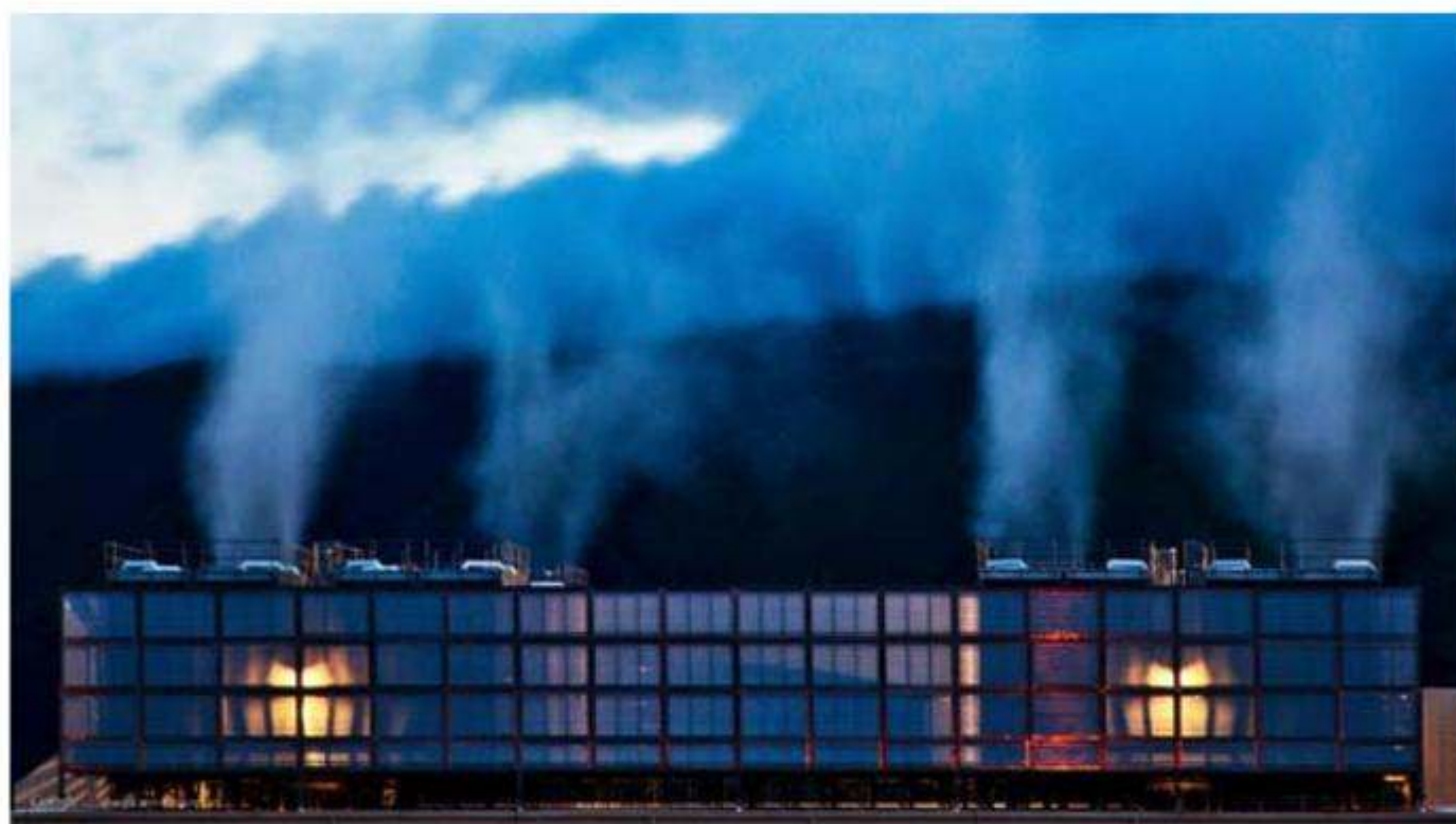
Figure 6.31 Steam rising from the cooling towers that transfer heat to the air from the water used to cool equipment.
