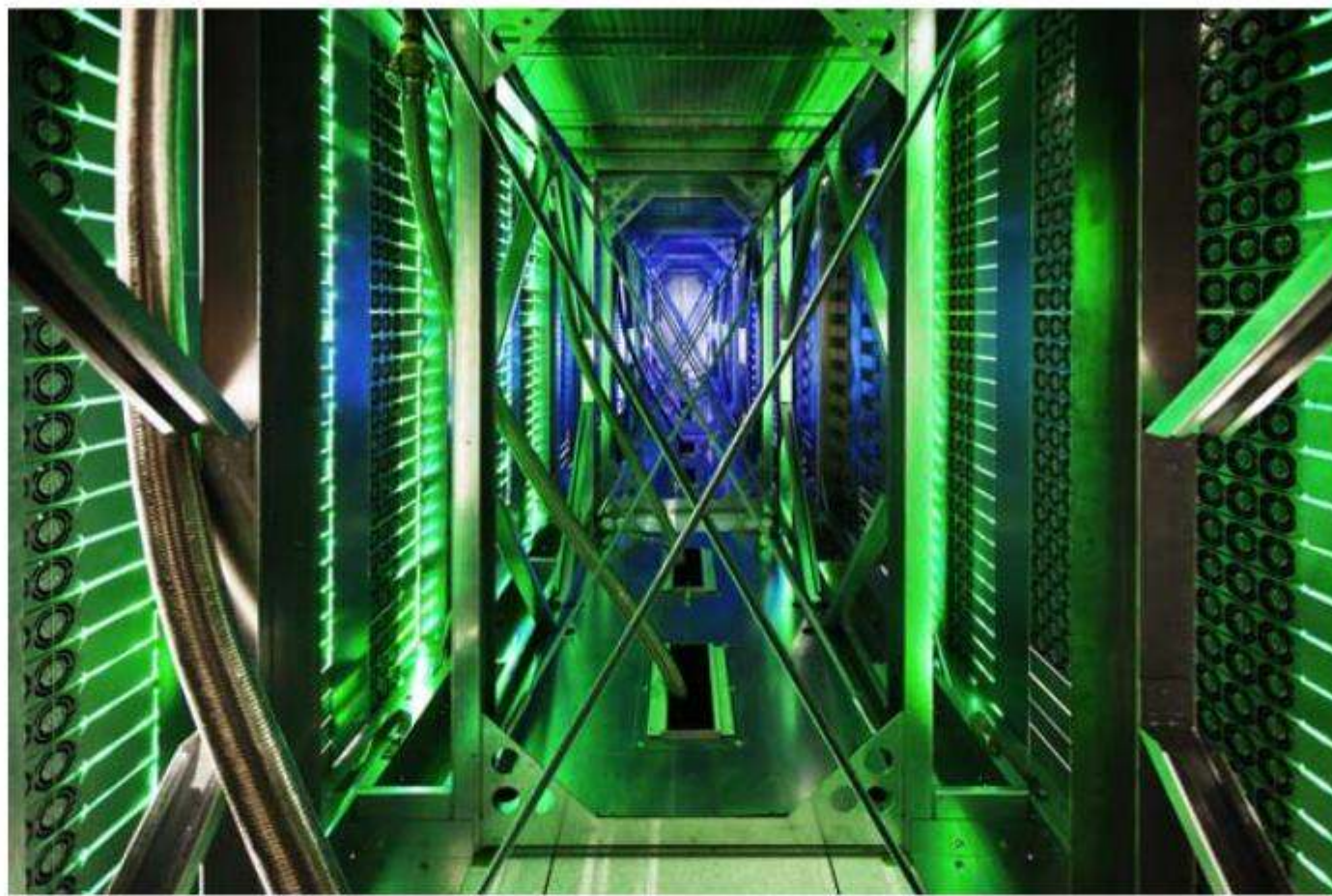
Figure 6.29 Hot aisle in a Google data center, which is clearly not designed to accommodate people.
